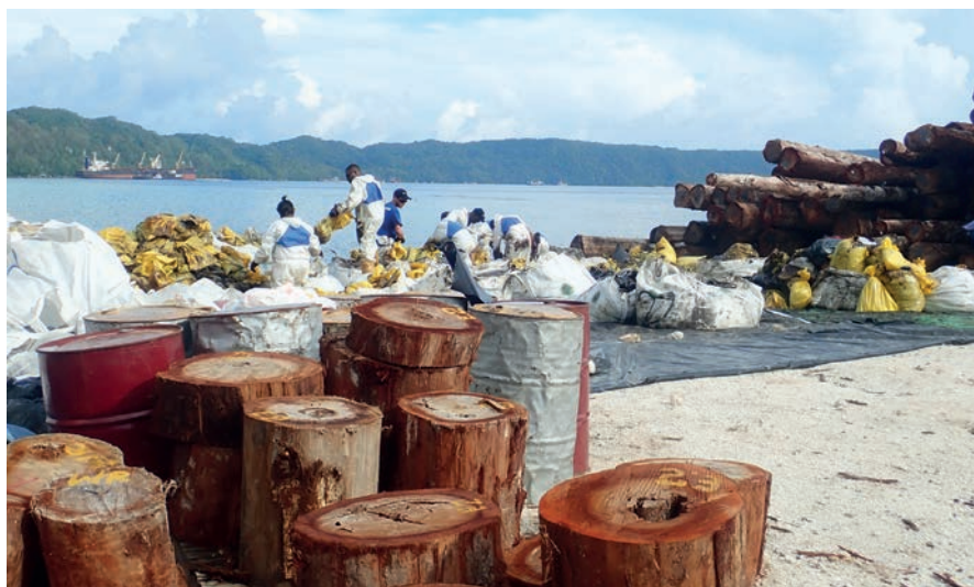
Temporary storage of oiled waste, Solomon Islands
