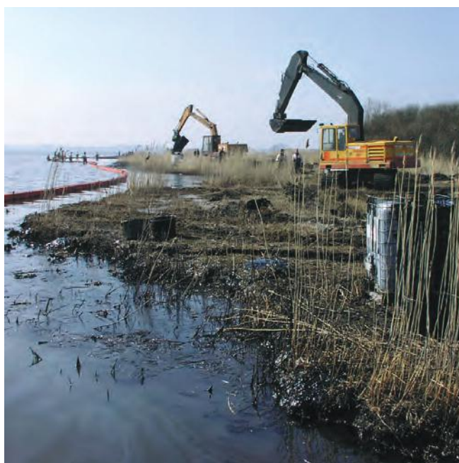
▲ Figure 41: Use of heavy machinery on sensitive areas of the shoreline may cause considerable additional damage. In this case, the need to rapidly recover free-floating oil was a priority.
