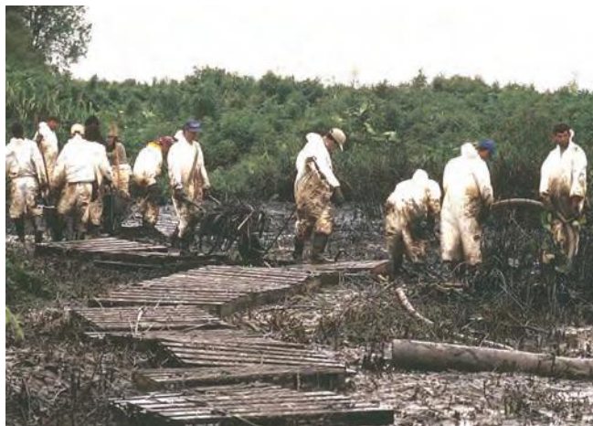
▲ Figure 40: Intrusive clean-up of an oiled marsh caused considerable additional damage over and above that of the oil itself.
