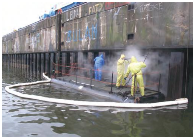
▲ Figure 30: Oiled pilings and dock quay being pressure washed from a small raft. Released oil is collected in the sorbent boom.
