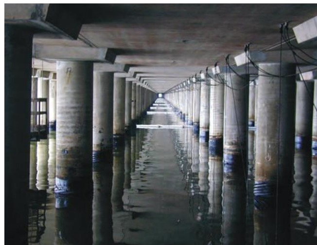
▲ Figure 5: Access underneath wharves may be difficult and dangerous for clean-up crews due to lack of head room and ventilation.
