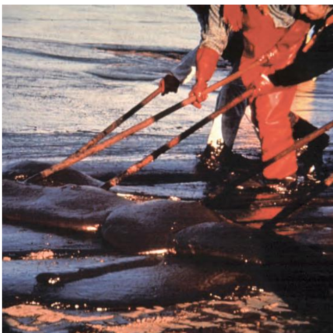
▲ Figure 12: Crude oil is scraped along a hard-packed sand beach to be collected in trenches and then recovered by vacuum trucks for onward transport to disposal.
