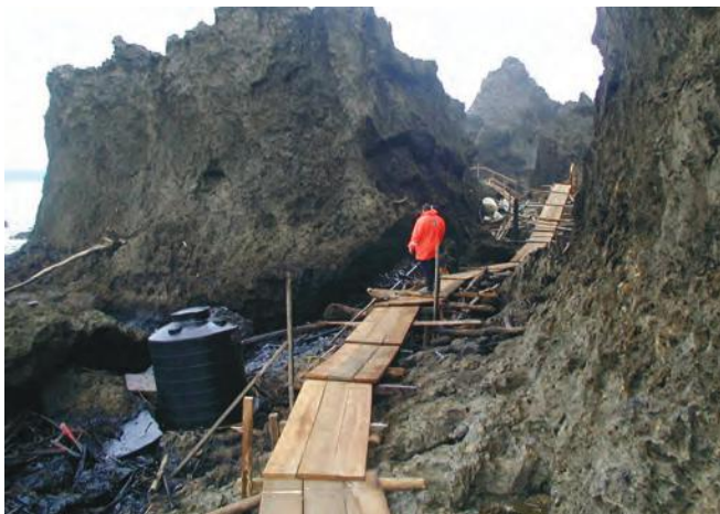
▲ Figure 35: To minimise hazards to workers on rocky shorelines, temporary walkways can be constructed.
